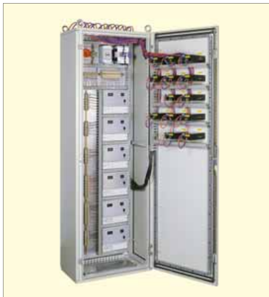
Internal view of the CMR Panel. An isolator, fuses, power supply, computer interface terminals and six DPC500 Controllers are fitted on the back plate. All factory tested.
