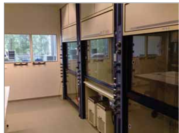
PFR-C Fume Hood Controllers in operation
